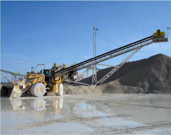
125' Fixed height radial stacker. This project started in early 2004 and ran through 2006. We replaced almost every conveyor in this plant including radial stackers, belt conveyors and feeders.
