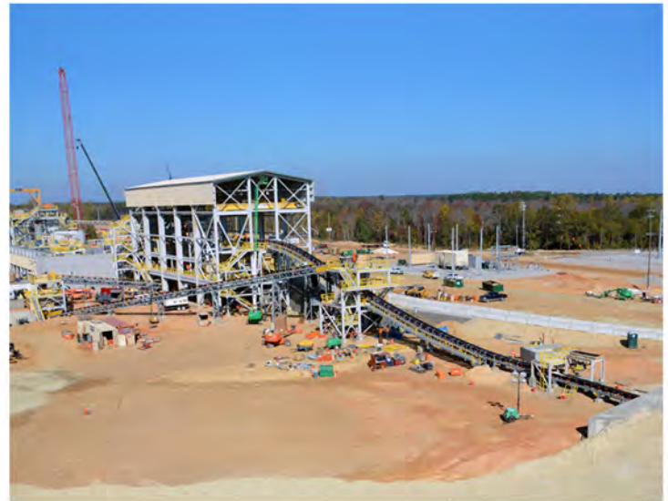
Completed in 2017, this particular gold mine is on the site of the longest continuously operating mine in US history. We provided five conveyors from primary crushing through the re-circulation circuit.
