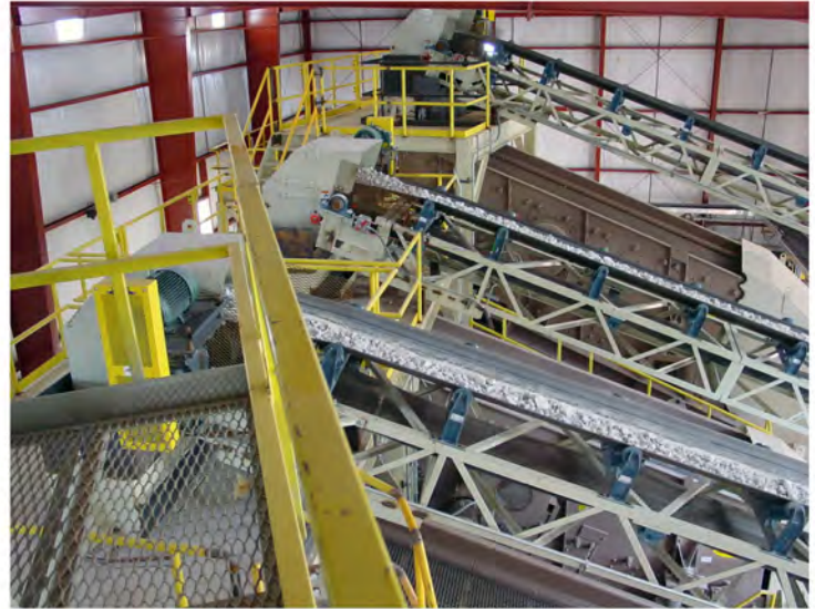
This was a unique job. The entire crushing and screening plant was enclosed in a metal building. A total of 26 conveyors were supplied on this project.
